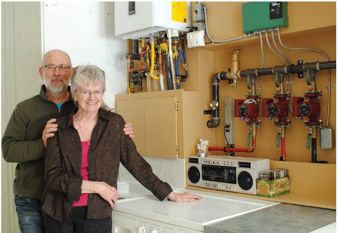
► Tom and Dee Ashman in the laundry room near the household mechanical systems that provide on-demand domestic hot water and back-up heat through in-floor heating.
